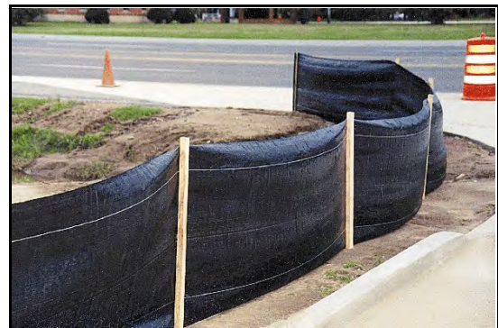
Silt fence and other perimeter controls far less effective than stabilization
