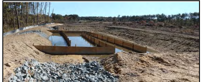
Perimeter Sediment Trap
